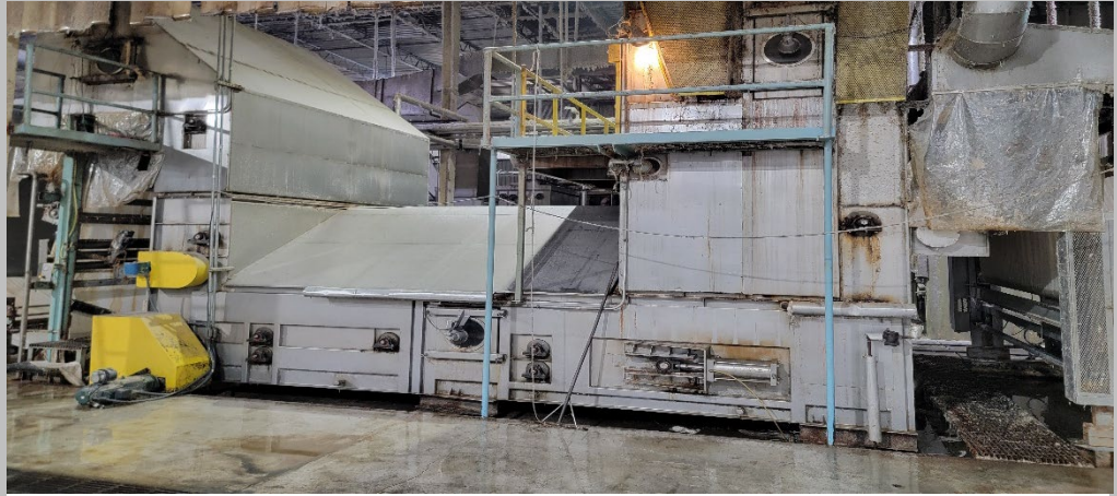
140" Wide Morrison 2-Stage Bleach Range No. 6 Steamer Unit
