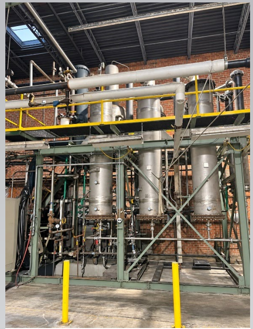
Three Stage Caustic Evaporator
